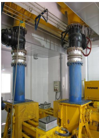
Photo: Sludge pump
